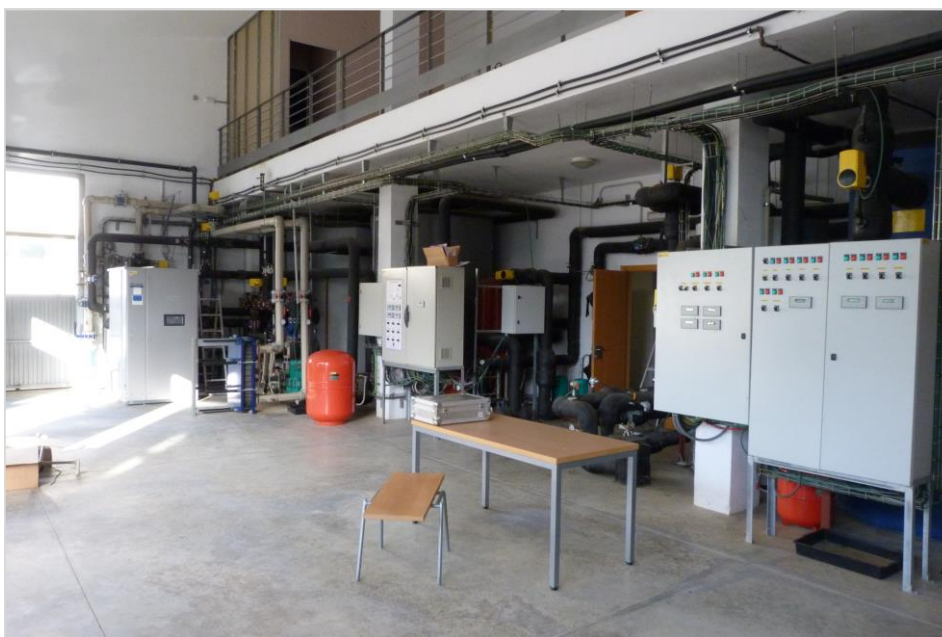
Solar cooling installation
