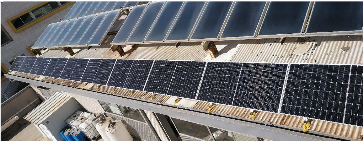
New photovoltaic modules for the CIESOL Smart-grid
