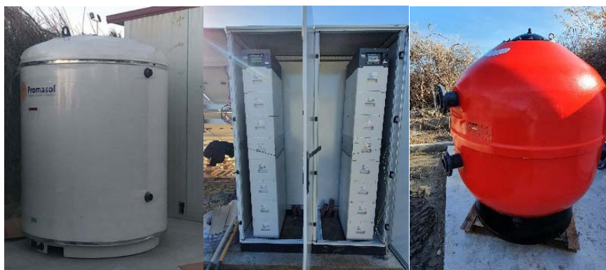
Thermal, electrical and CO2 storage tanks
