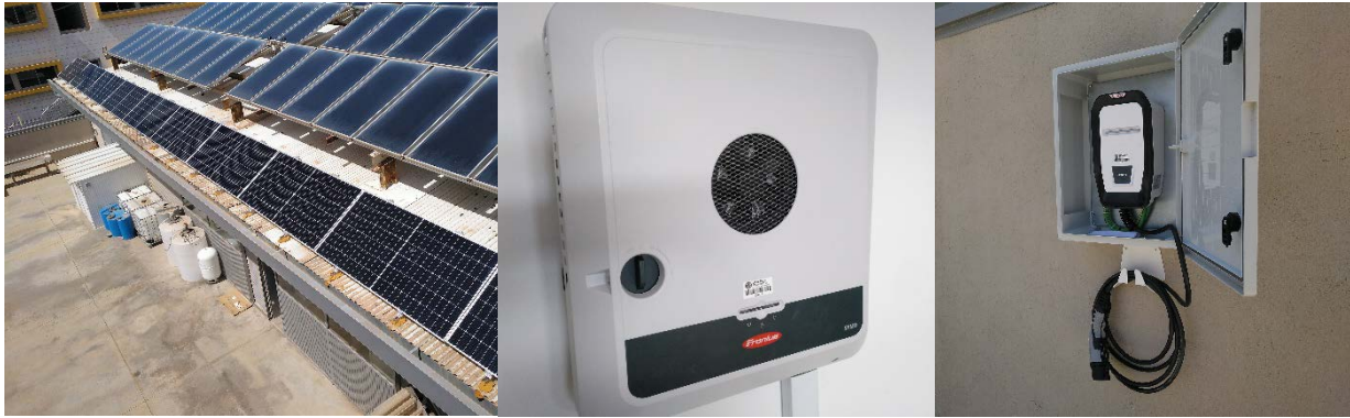
Photovoltaic modules, inverter-charger and electric vehicle recharging point
