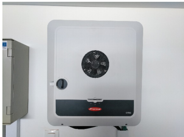
New advanced inverters
