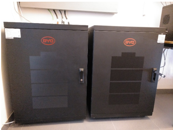
Lithium batteries for electricity storage
