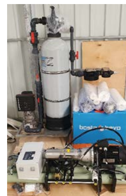
Reverse osmosis plant
