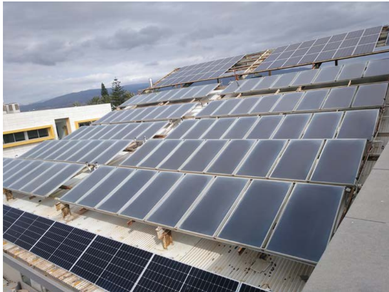
Solar collector field
