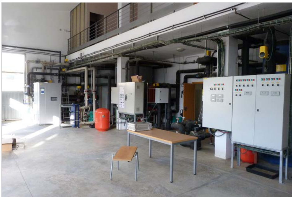
Solar cooling instalation
