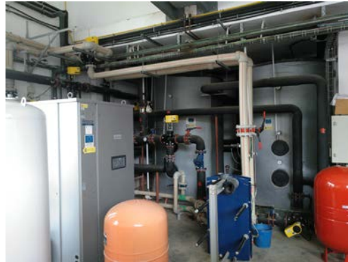
Yazaki absorption machine and hot water storage tanks
