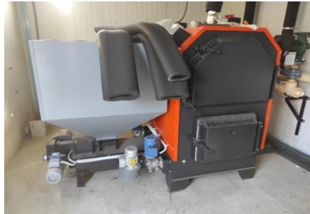
Thermal conditioning system
