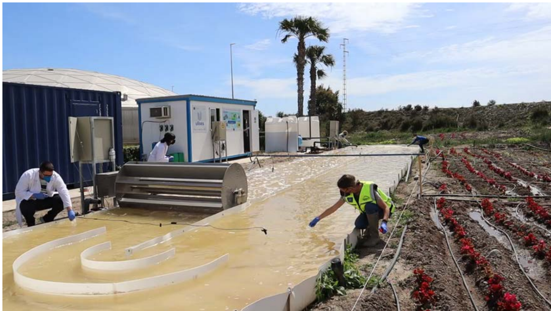
Figure 2.3.1. Raceway pond reactor for the operation of the solar photo-Fenton process in continuous flow mode for the treatment of secondary effluent, installed at the “El Bobar” WWTP in Almería.
