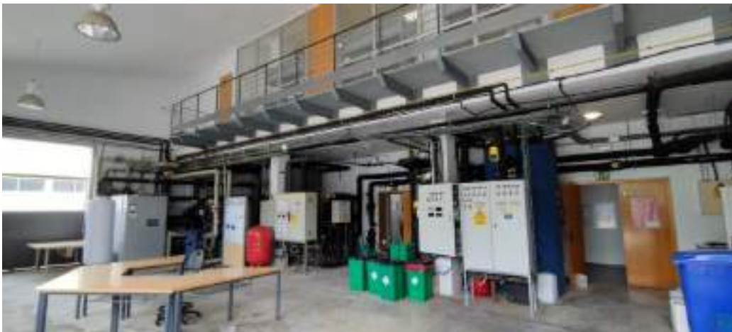
NAVE CIESOL – Solar cooling installation
