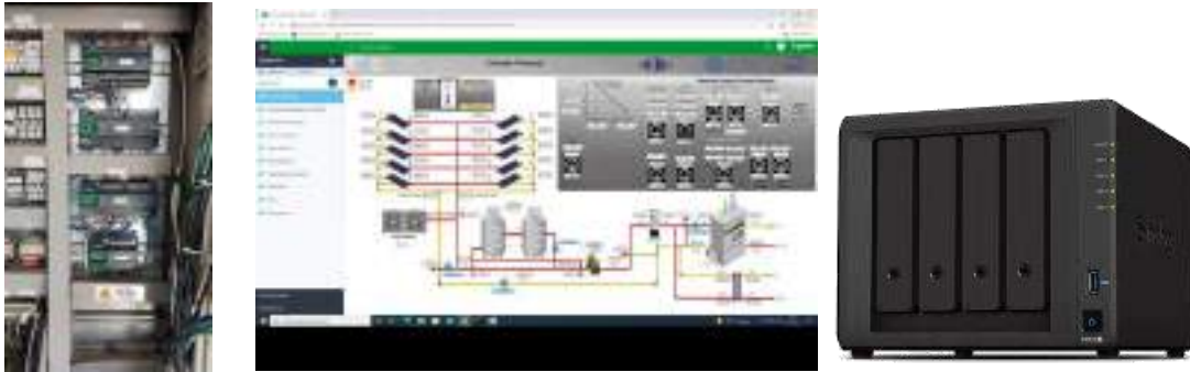
PLCs of Schneider Electric. New acquisition application and server to store the data.
