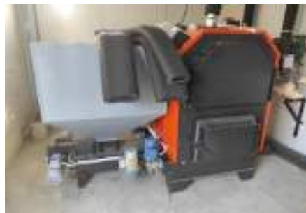
Thermal conditioning system
