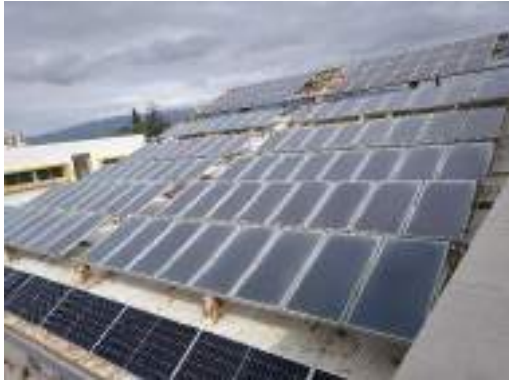
Solar collector field
