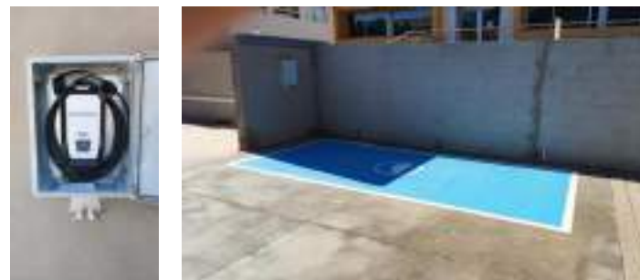
Charging point for electric vehicles
