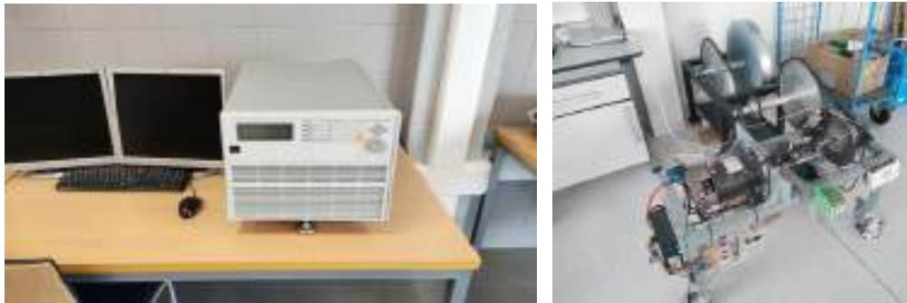
Load simulator (left). Charging station for electric vehicles (right)
