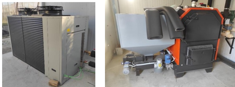
Thermal conditioning system
