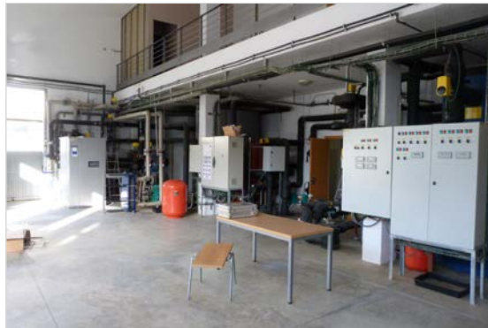
NAVE CIESOL – Solar cooling installation
