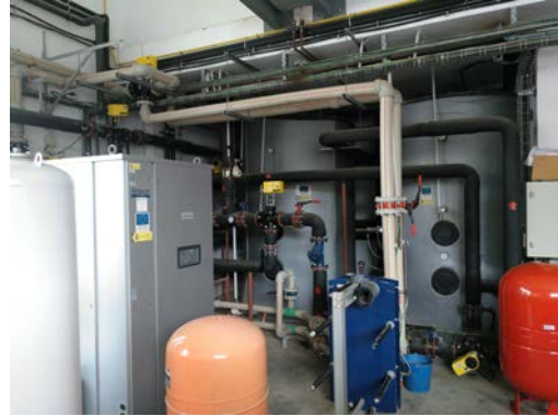
Yazaki adsorption machine and hot water storage tanks
