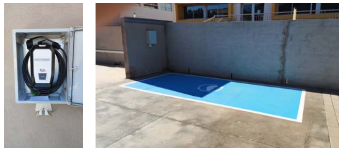
Charging point for electric vehicles
