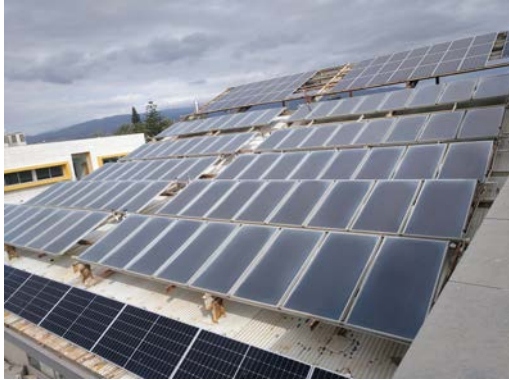
Solar collector field
